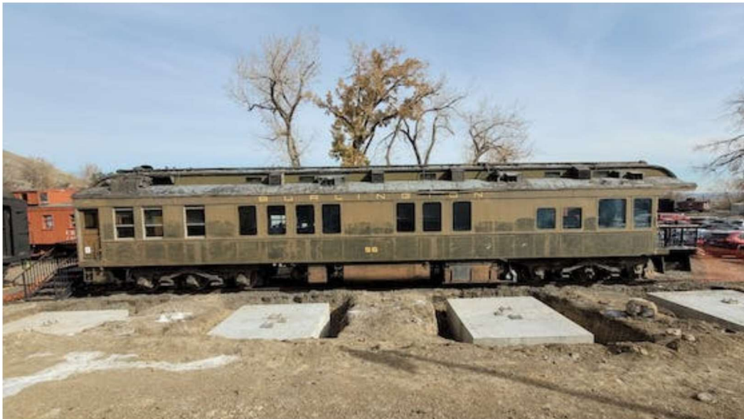
The Colorado RR Museum will soon be erecting a cover that will give some weather protection for displayed rail cars. The base concrete blocks are seen here next to CB&Q business car #96 on 12 Nov 2022. ©2022 Dave Schaaf
